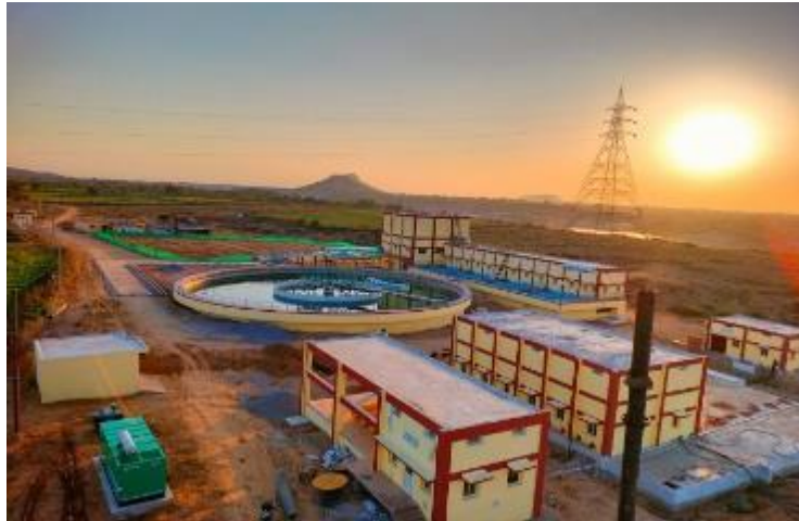
24 MLD Lahchura Water Supply Scheme in Uttar Pradesh under Jal Jeevan Mission of Central Govt.
