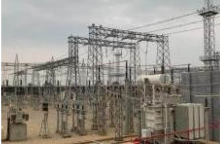
220/132 kV Substation in Botswana
