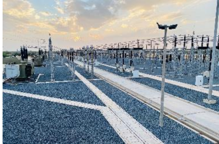
225/30 kV Substation in Senegal
