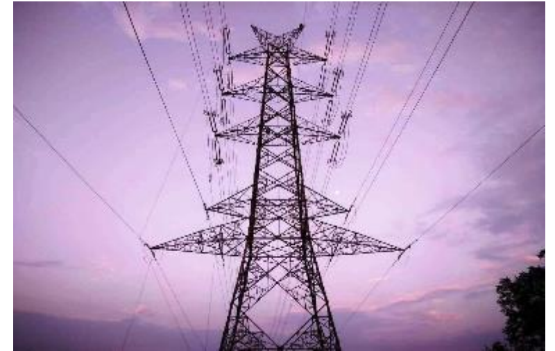
765 kV D/C 190 Km Transmission Line in Uttar Pradesh, India
