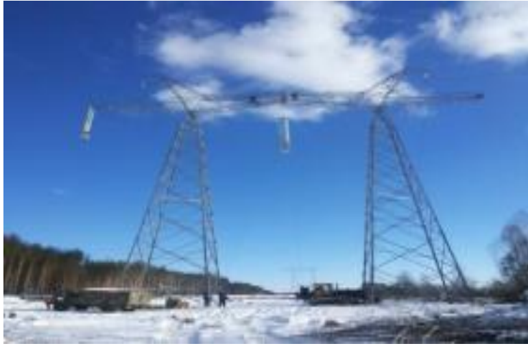
750 kV S/C 353 Km Transmission Line in Ukraine
