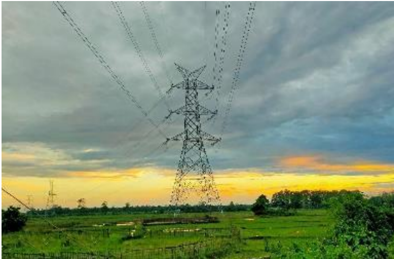
400 kV S/C 112 Km Transmission Line in South Africa
