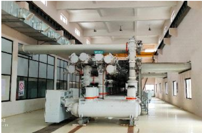
400 kV GIS Substation in India
