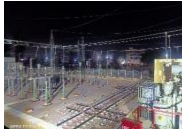
Daliganj-Kasganj Railway Electrification
