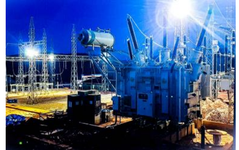
220/30 kV Substation in Burundi
